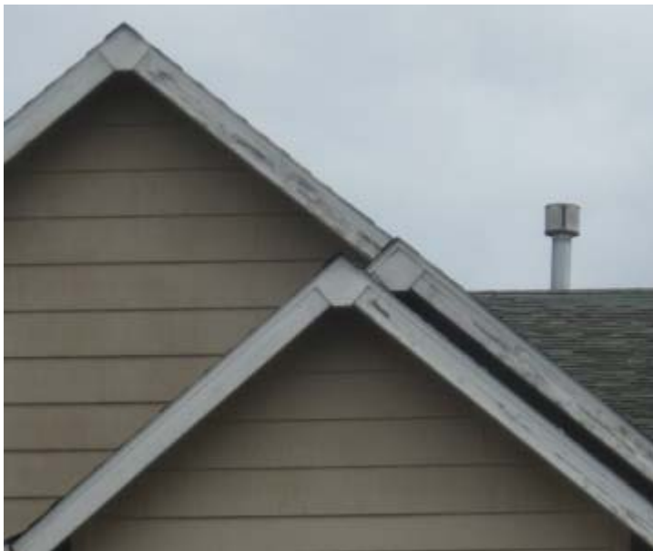
Trim paint is faded and peeling
